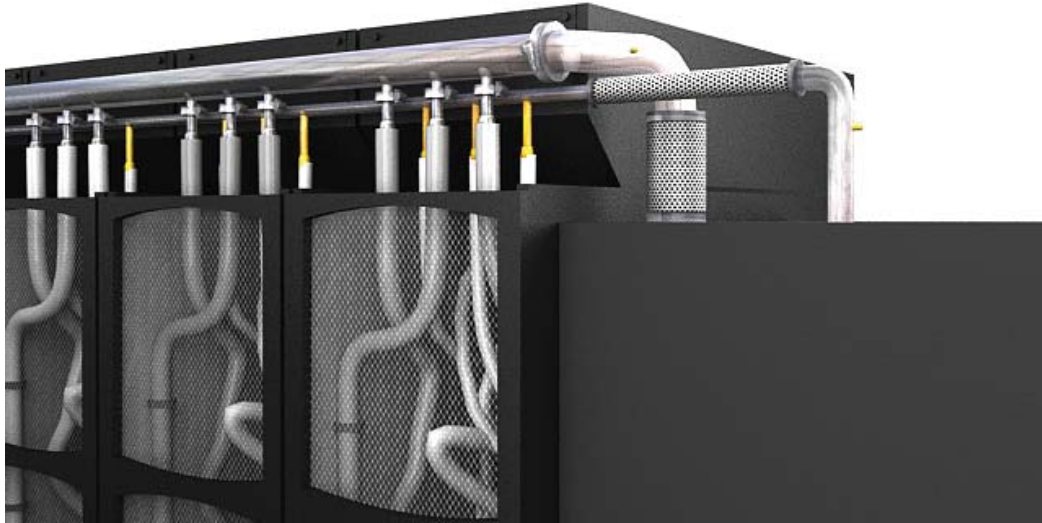
Figure 7.6: An example of plumbing in a liquid-cooled system (source Cray Inc.).
