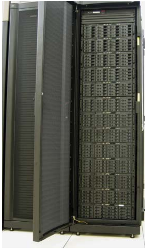
(a) 19-inch rack.
